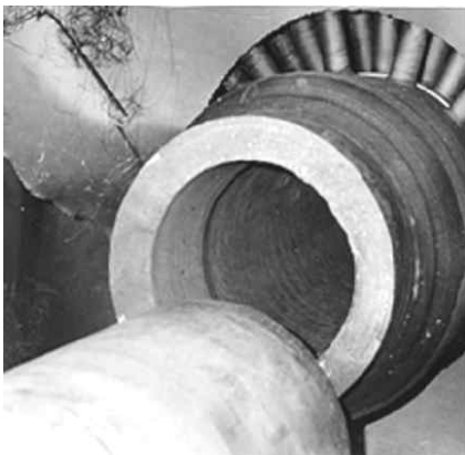
Fig. 1 Example of weld section cutting damage by residual stresses in main steam pipe of power plant
