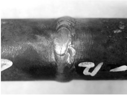
Fig. 1 Appearance of weld metal reheat crack developed in the form of through-crack
